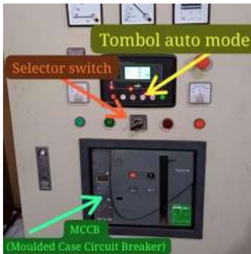
Gambar 4.2 Panel Control Genset
