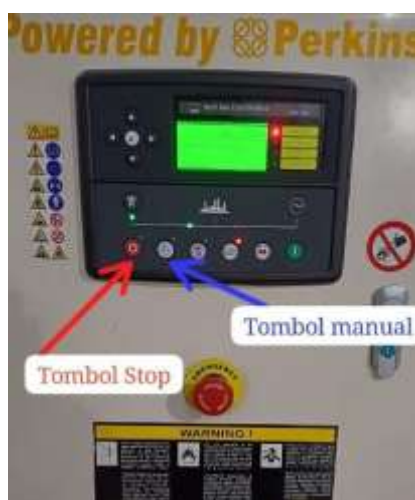
Gambar 4.3 Panel Control Genset
