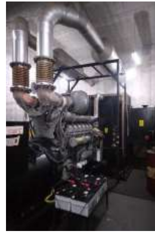
Gambar 4.1 Generator Set (genset)
